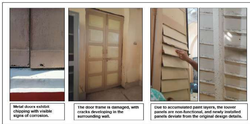
Figure 11: Problems arising in the current doors and openings.
