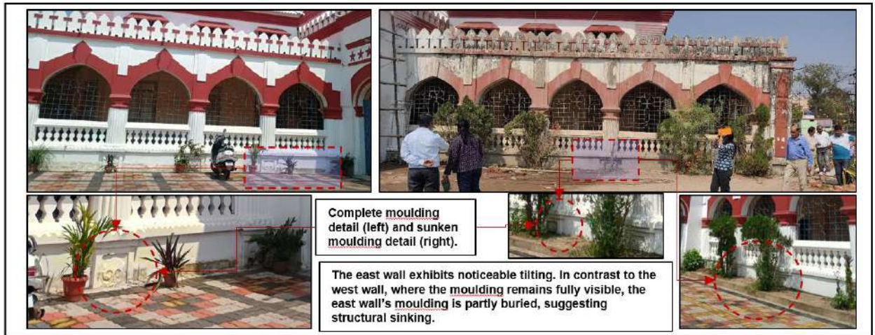
Figure 3: Structural settlement of east wall
