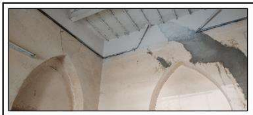
Figure 4: Cracks in the walls
