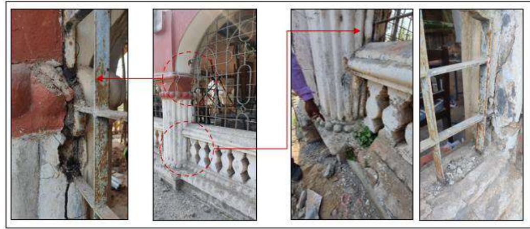
Figure 14: Corrosion of metal grill causing cracking in the adjoining wall
