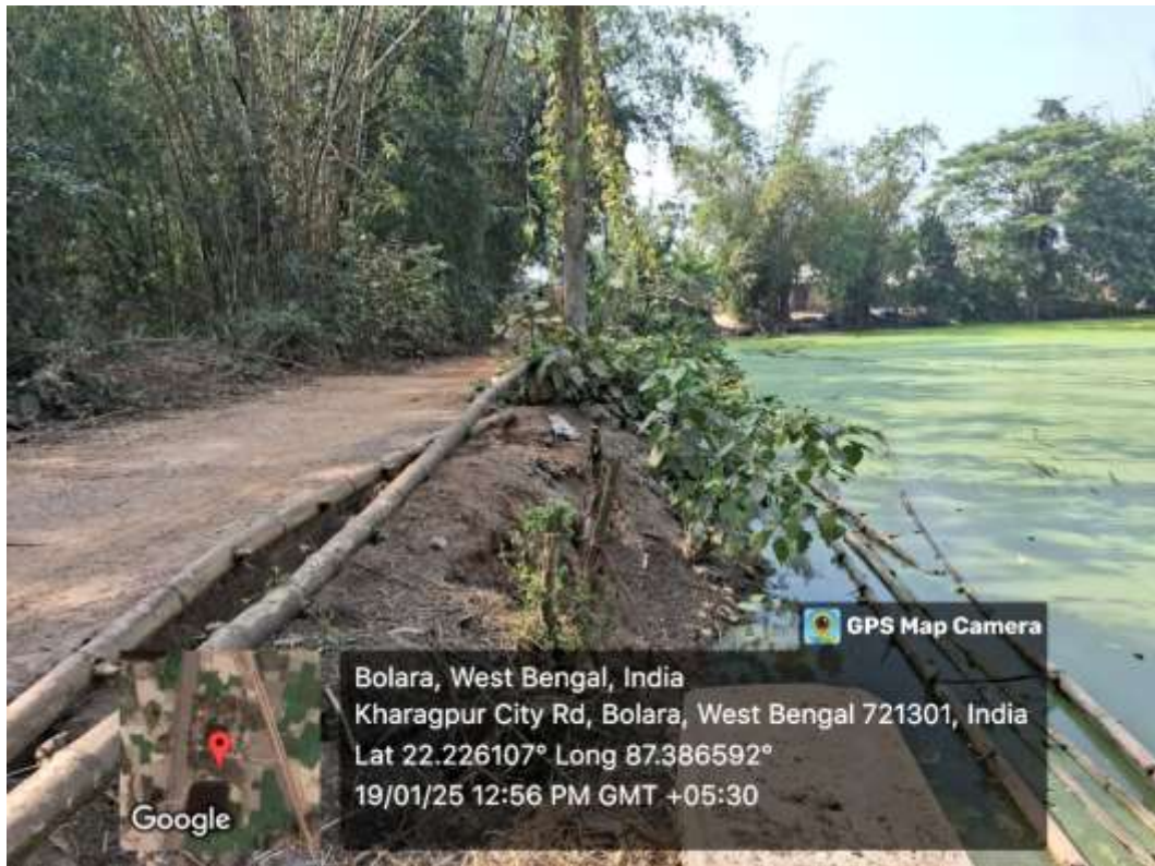
Figure 3-47 Absence of guard wall around the pond
